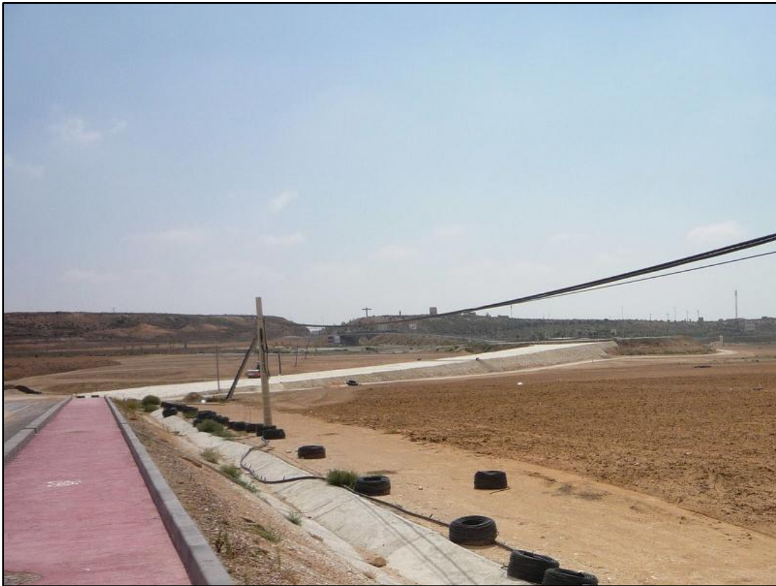
New road to Sucina – base for the road embankment to the level of roundabout now constructed
